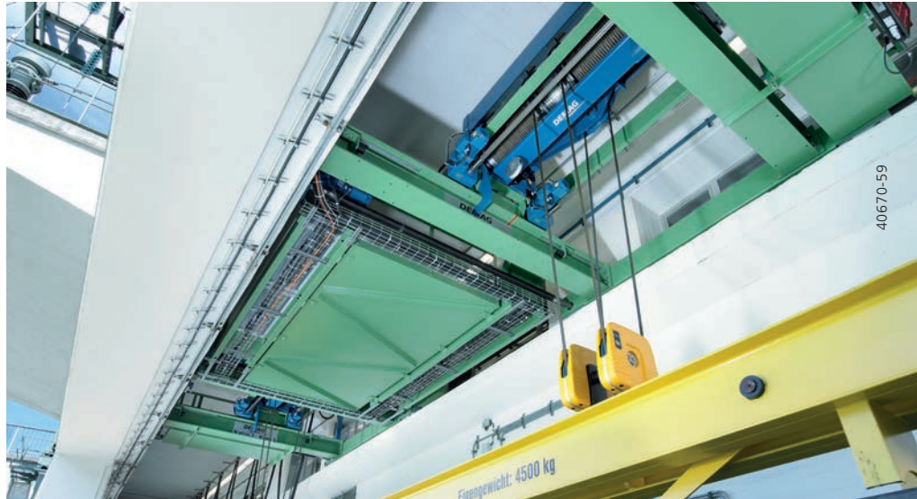
Dam beams are positioned with 2 DH hoist units at water depths of up to 22 m.
