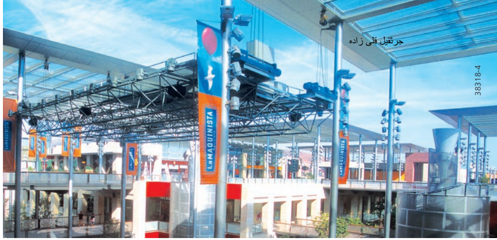
Lifting and lowering a steel and glass roof structure with 4 DH hoist units
